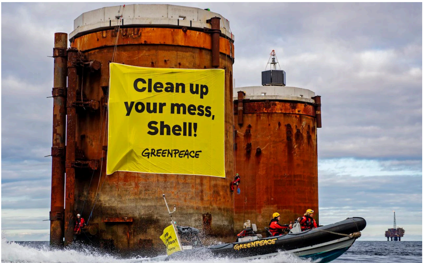
Ageing oil rig structures left to rust in the North Sea have infuriated environmental groups | CREDIT: Greenpeace
